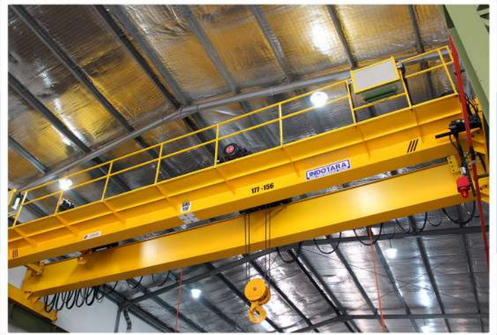
OVERHEAD CRANE DOUBLE GIRDER
