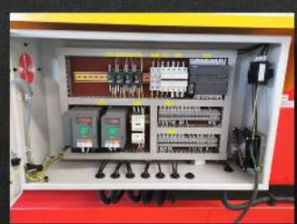
Schneider frequency inverter
