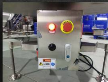
Control Box Panel
