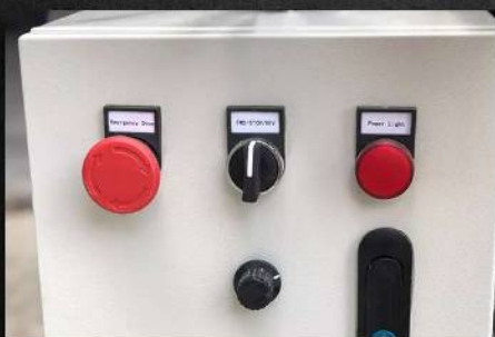
Control Panel Forward, Stop, Reverse, Adjust Speed
